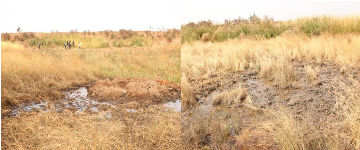
Figure 5: Water Oozing from the Ground Behind the Vunania Dam
