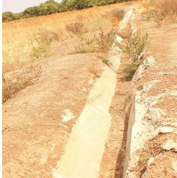
Figure 7: Canals in the Vunania Irrigation Area Showing Defective Construction
